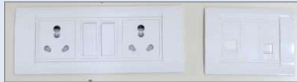
▲ INBUILT SWITCHES, SOCKETS, LAN AND TELEPHONE CONNECTIONS
